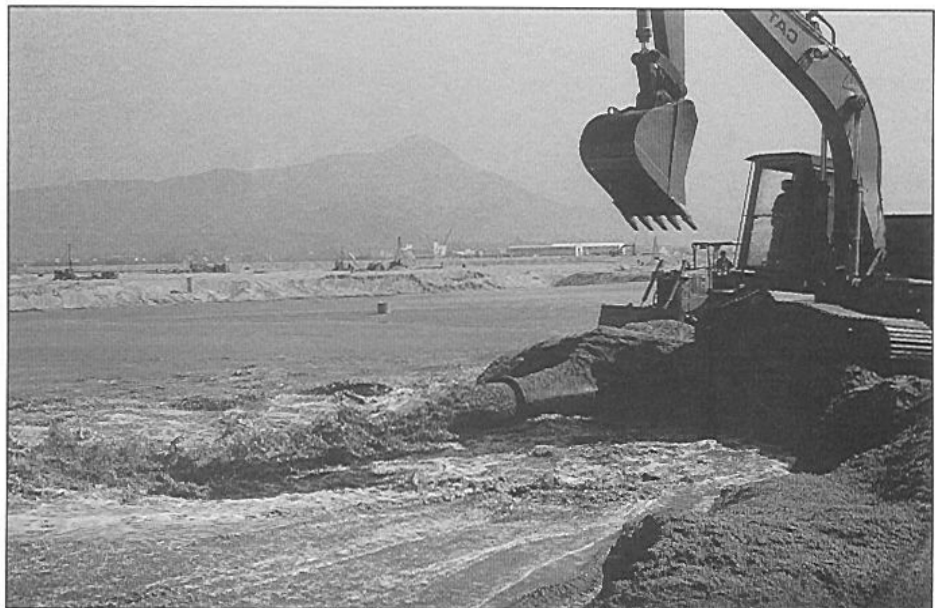
Plate 4 - Placing marine-dredged sand in the Tin Shui Wai Reclamation in Junk Bay
