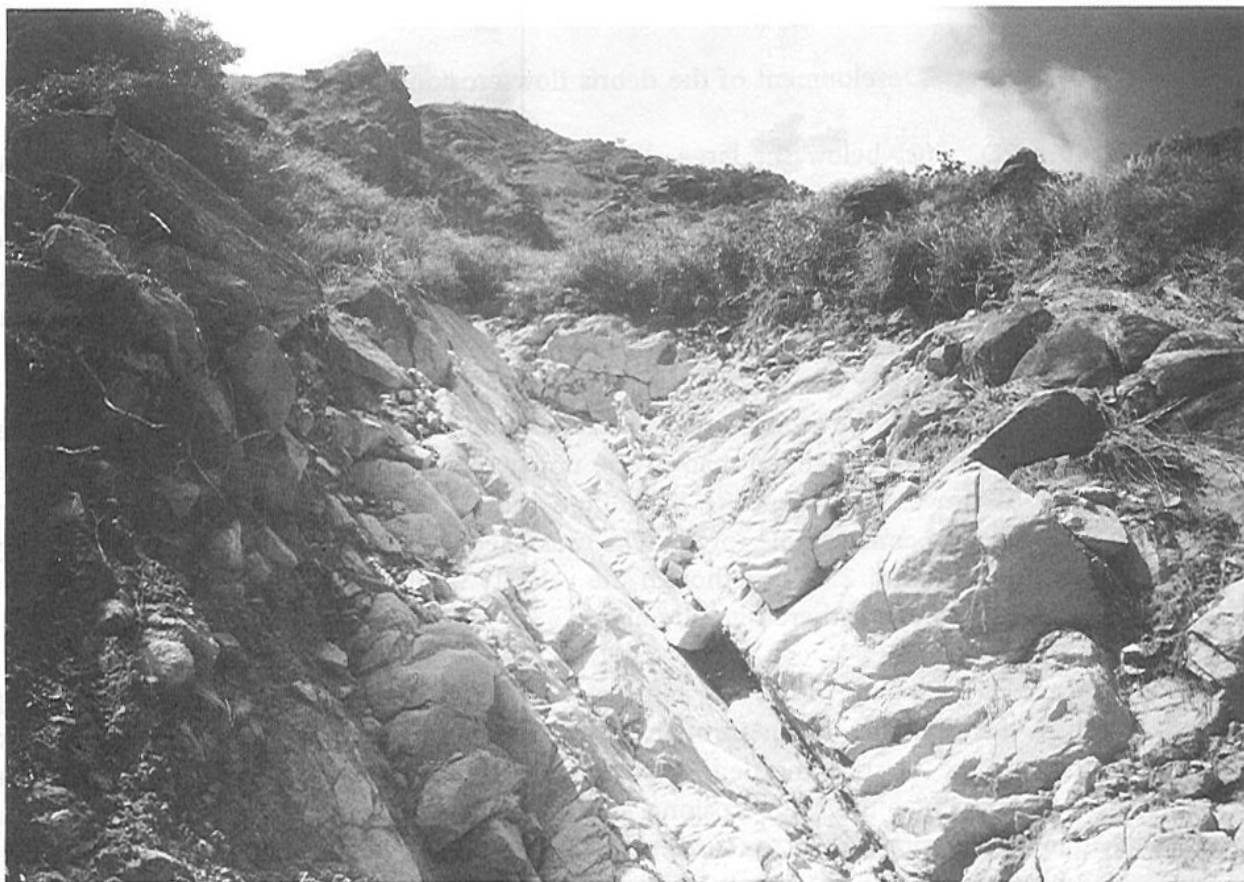
Plate 2 V-shaped channel immediately below the initial failure, with freshly exposed granite bedrock; note one of the authors standing in front of the rock overhang
