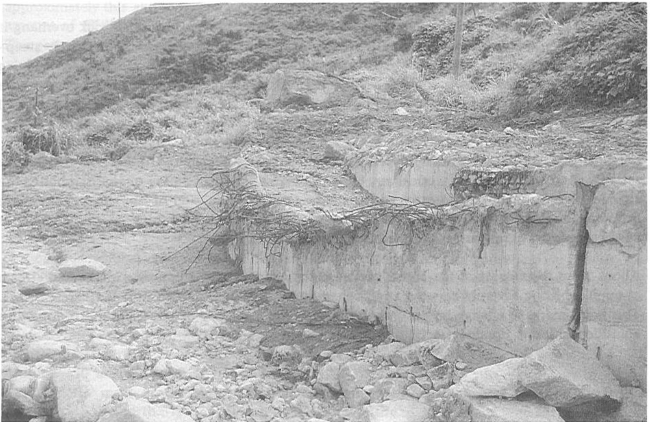
Plate 5 Abraded and broken concrete stream intake at the top of the depositional area
